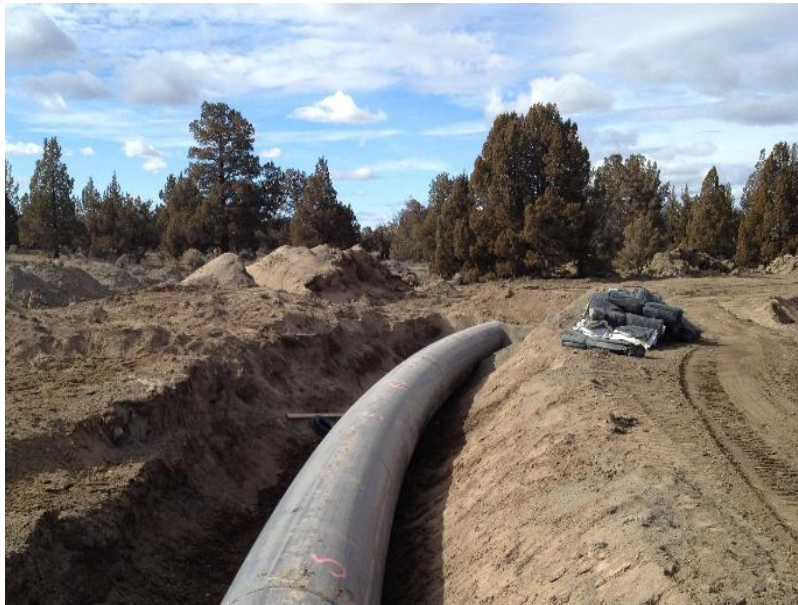
The I-Lateral was one of the leakiest canals in Central Oregon Irrigation District.
